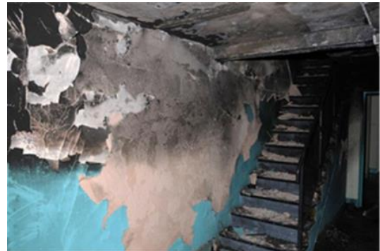
Stairwell opposite the scooter. Note: spalled plaster from the stairwell has fallen onto the stairs
