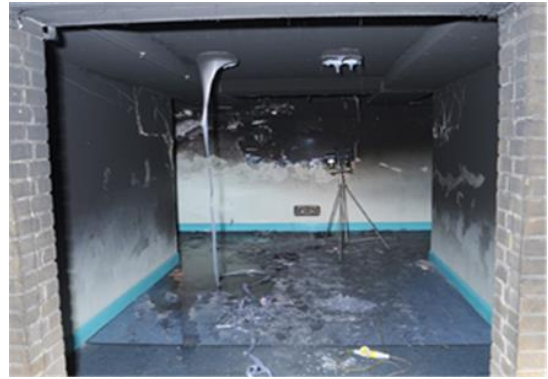
entrance. Note light fittings have melted
