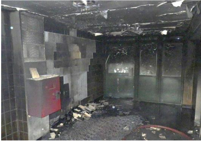
Image left: View of communal area with the remains of the mattress in foreground. Note damage to ceiling and walls, doors and wall panels.
