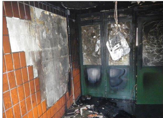
Image right: View from other side of doors. Note extensive damage to ceiling, walls, doors and wall panels. Light fitting and electrical wiring indicated by red arrow also damaged by fire.
