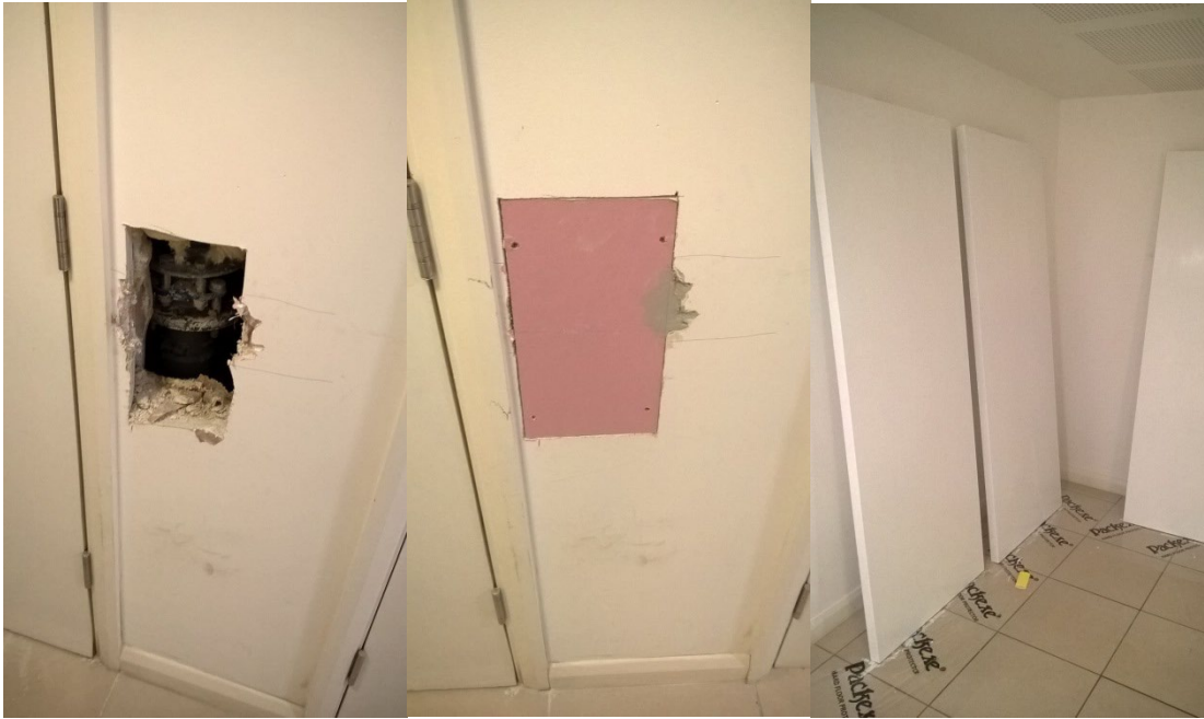
Damage from initial audit
