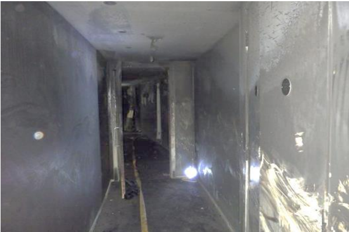
Images showing the 8 th floor corridor looking towards the flat of origin
