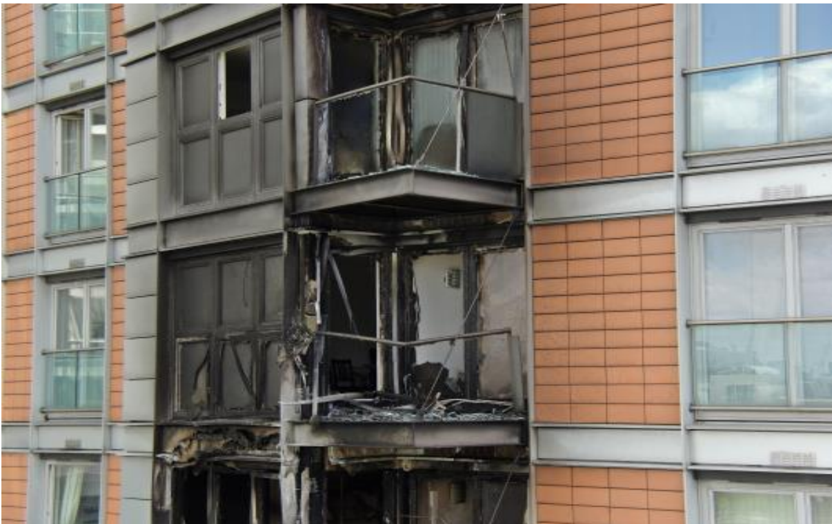
Image showing the external fire damage on the 9 th and 10 th floors
