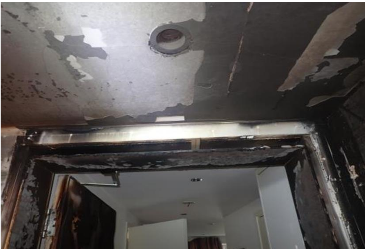
Image showing the void between the top of the door frame and the fabric of the building
