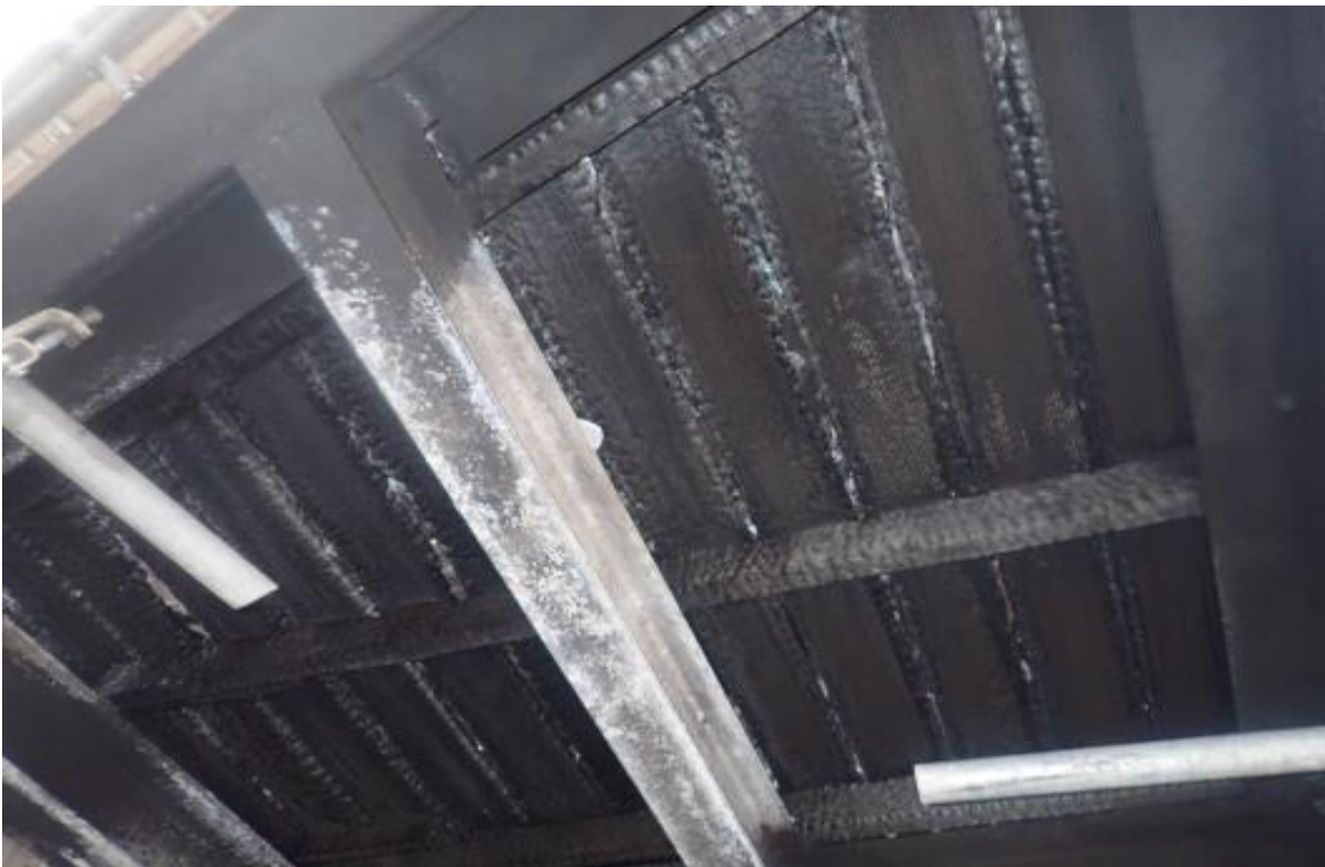
Image showing the charring to the underside of the 9 th floor balcony timber decking
