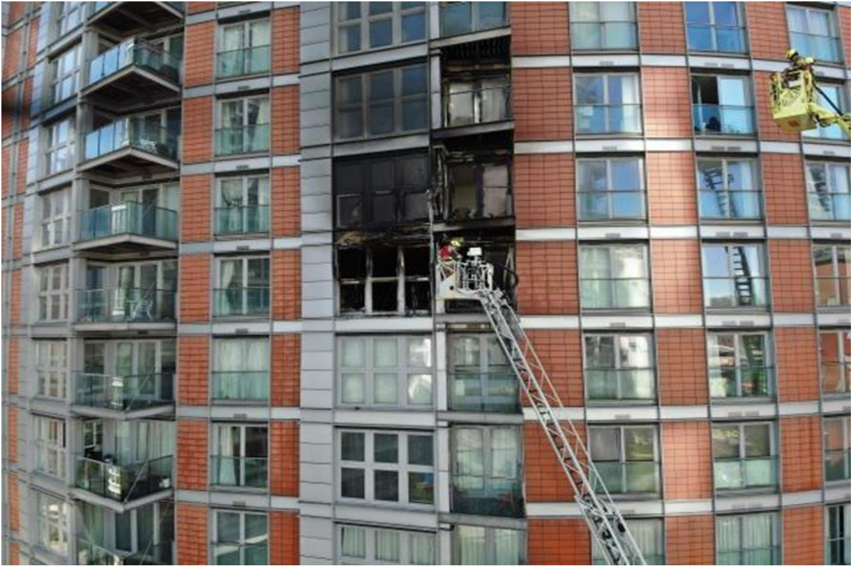
Images showing the damage to the exterior North face of NPW
