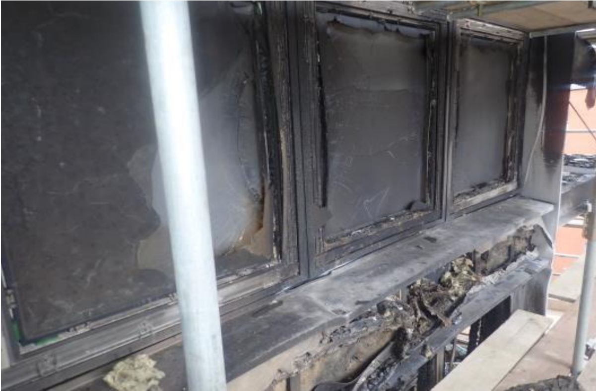
Image showing the damage to the ACM cladding between the 8 th and 9 th floor windows
