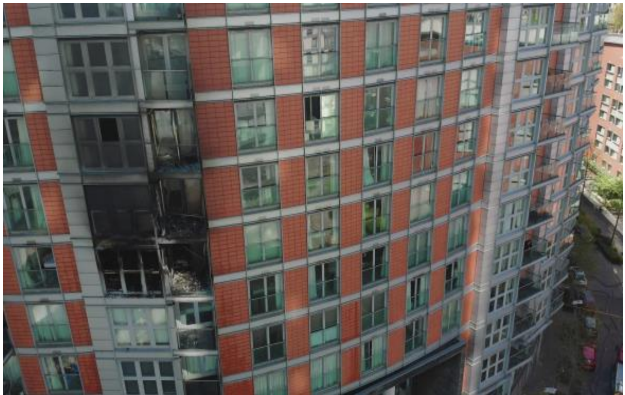
Images showing the damage to the exterior North face of NPW
