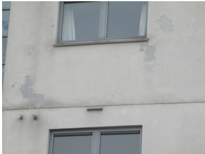
23 – Typical location where the render is failing.
