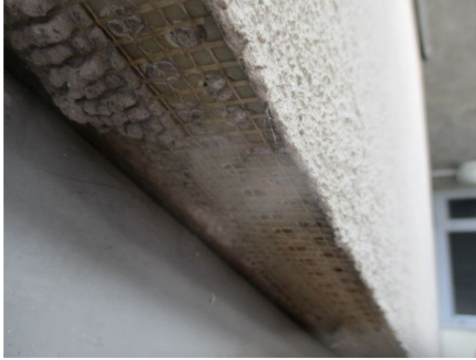
16 – Location 6 – Insulation exposed beneath panel
