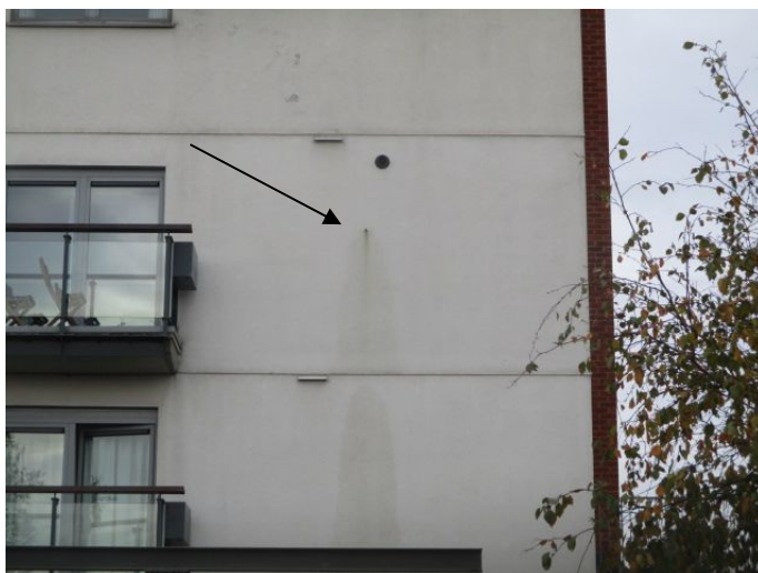
25 – Typical unsealed pipe through render.
