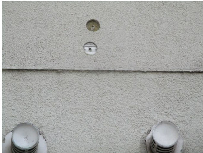
11 – Location 4 – Horizontal rockwool barrier
