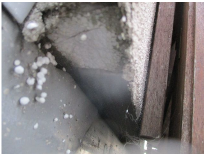
21 – Location 10 – Polystyrene insulation exposed at base of panel
