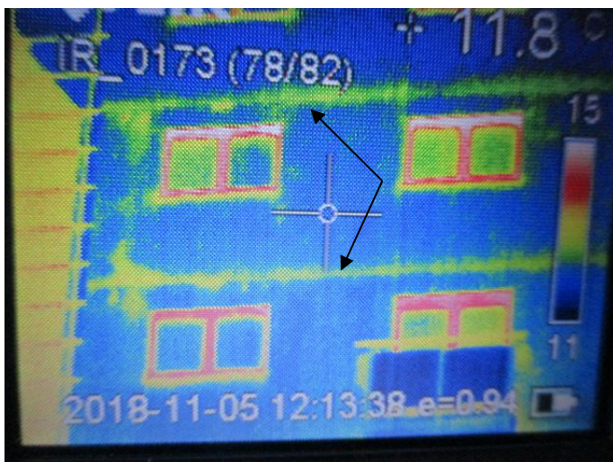
27 – Typical thermal anomalies at slab level (possible cavity/fire barriers ?).
