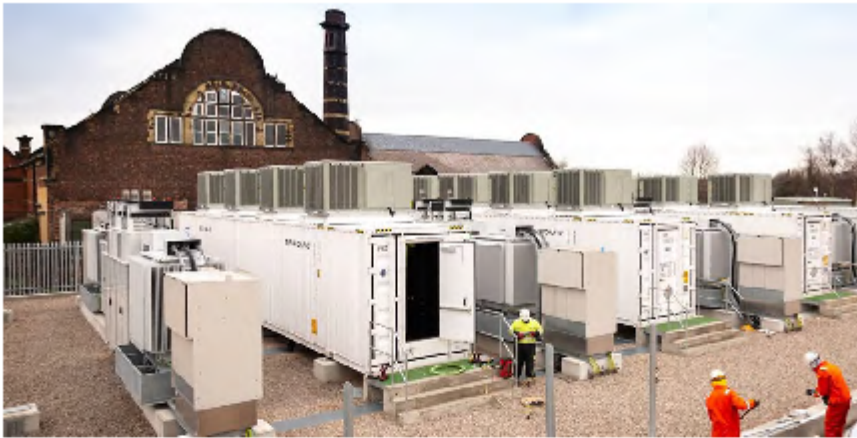
Figure 5 LiBESS installation on Merseyside that exploded in September 2020
