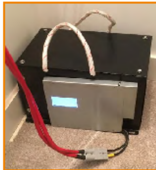
Figure 2 DIY domestic BESS
