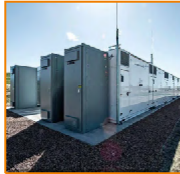
Figure 3 Industrial scale BESS
