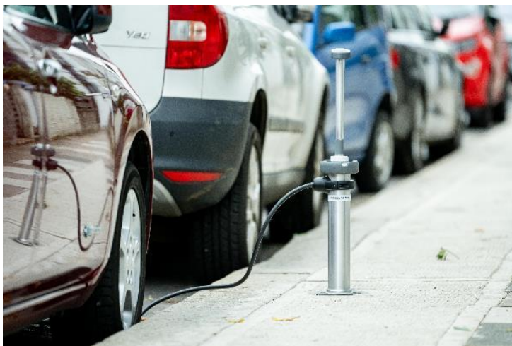
Figure 12: Pop-up charge points, Image courtesy of Trojan Energy Ltd
