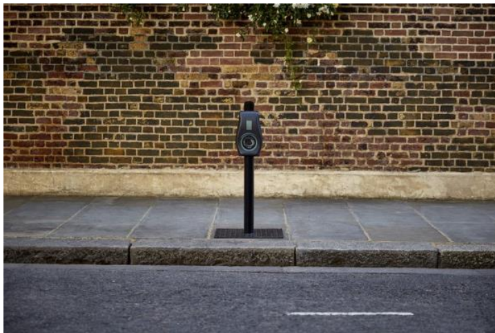
Figure 10: Gecko charging point by Connected Kerb
