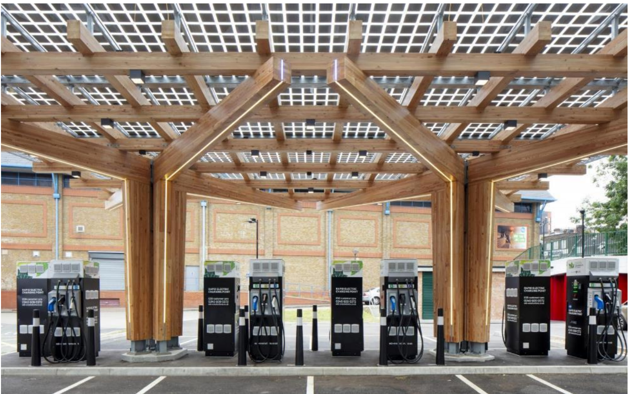
Figure 24: Glass Yard rapid charging hub
