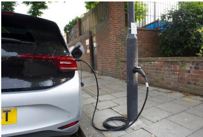
Figure 9: Lamp post charge point, Source: Ubitricity (member of the Shell Group)
